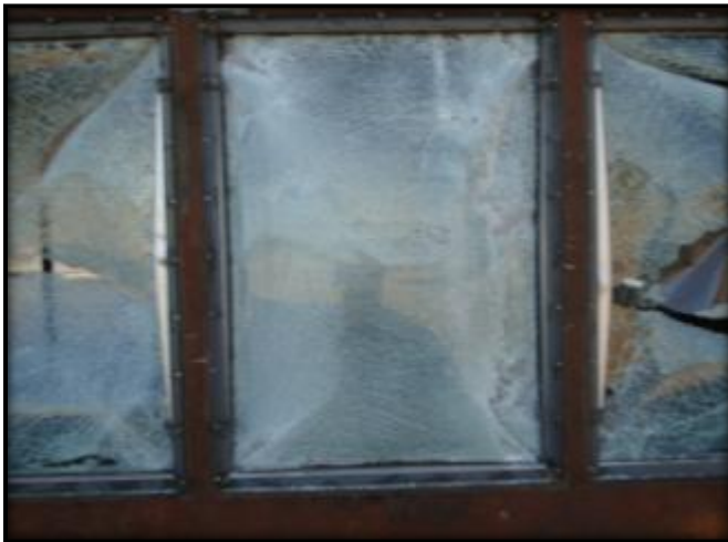
Figure C.31: L7 External Post-Blast Condition
