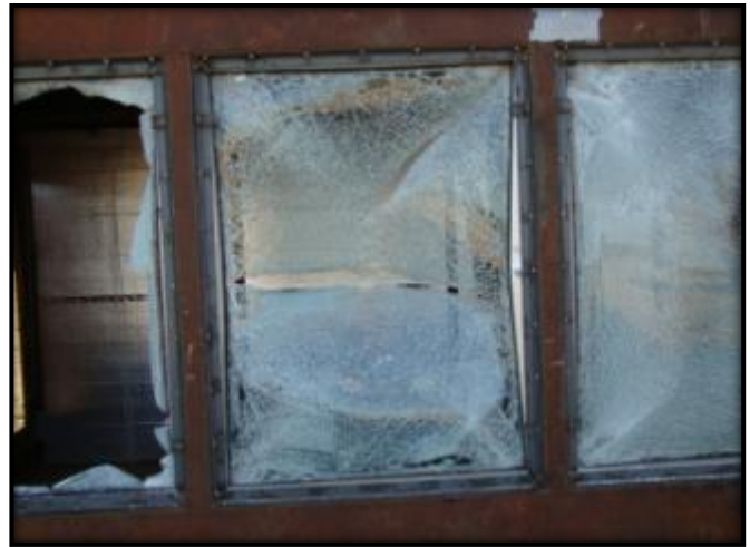
Figure C.30: L6 External Post-Blast Condition
