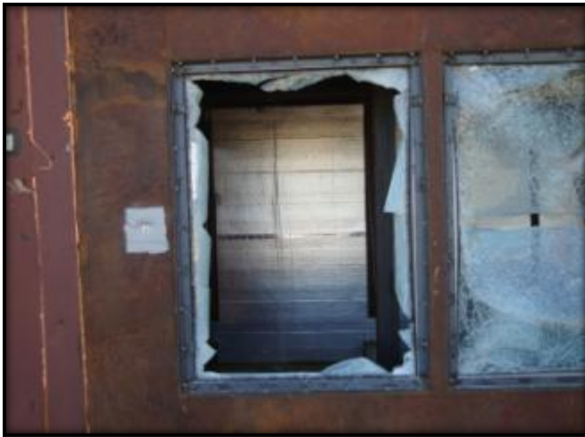
Figure C.29: L5 External Post-Blast Condition
