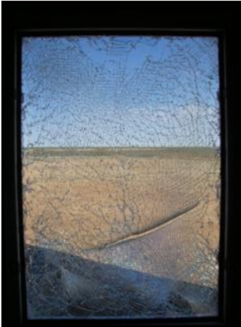
Figure C.13: L2 Internal Post-Blast Condition
