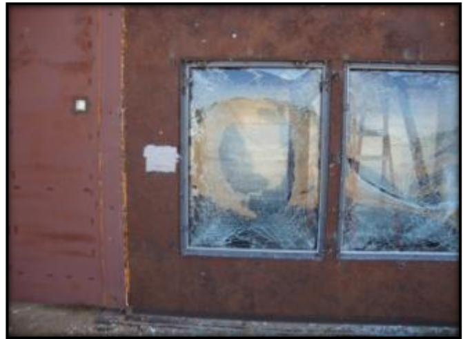
Figure C.8: L1 External Post-Blast Condition
