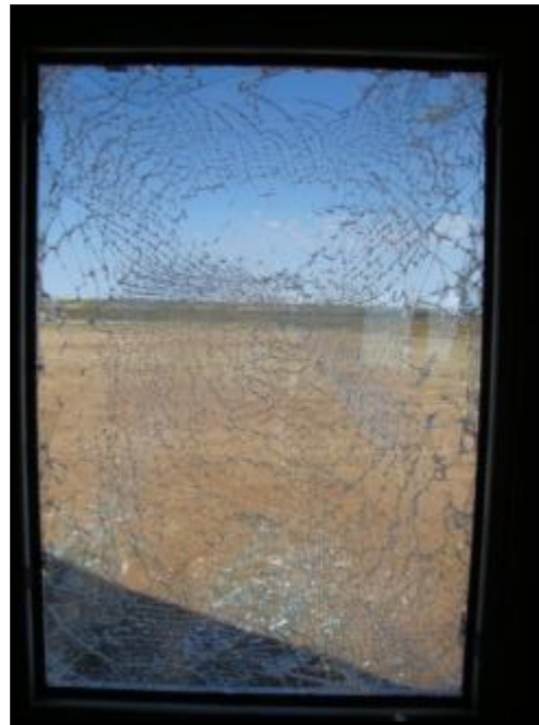
Figure C.12: L1 Internal Post-Blast Condition
