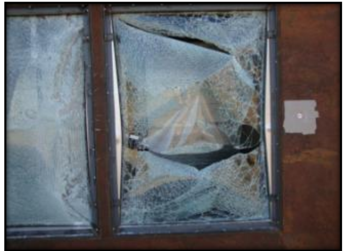
Figure C.32: L8 External Post-Blast Condition
