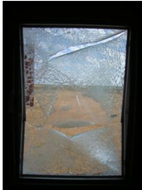
Figure C.36: L8 Internal Post-Blast Condition
