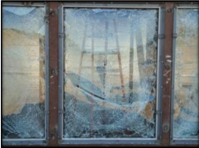
Figure C.9: L2 External Post-Blast Condition
