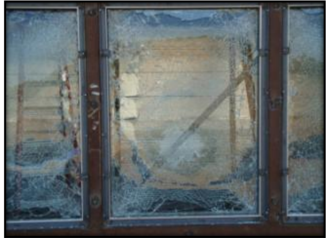
Figure C.10: L3 External Post-Blast Condition
