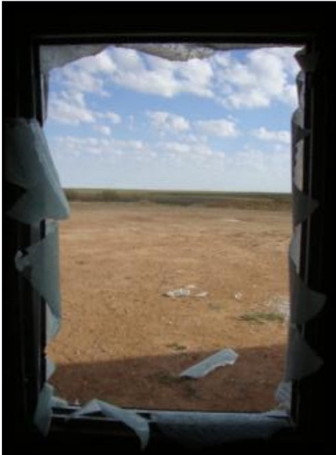
Figure C.33: L5 Internal Post-Blast Condition
