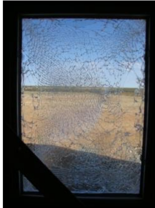
Figure C.14: L3 Internal Post-Blast Condition
