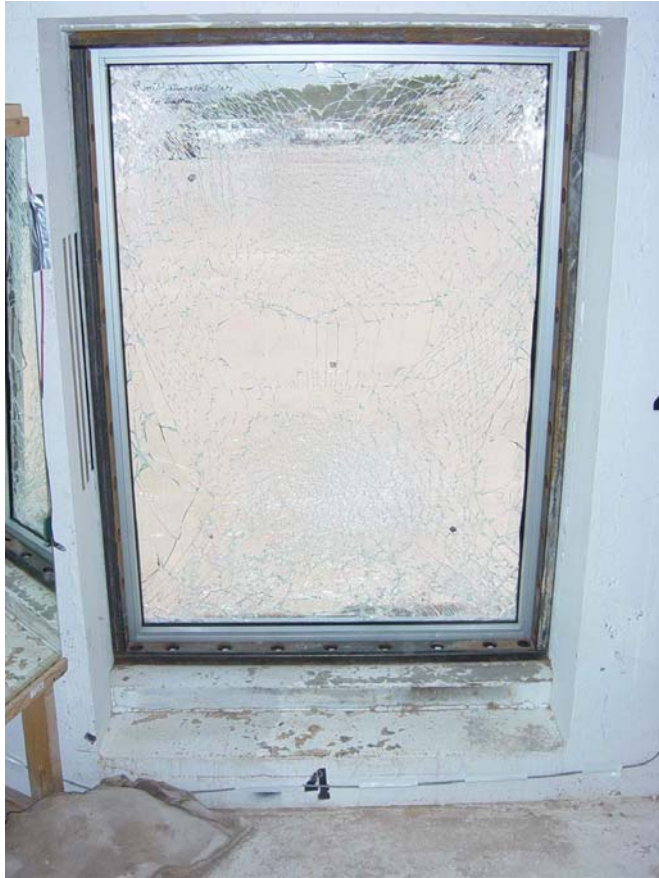
Figure 3-52 Interior post-test view of window 4. (DSC04432.jpg)
