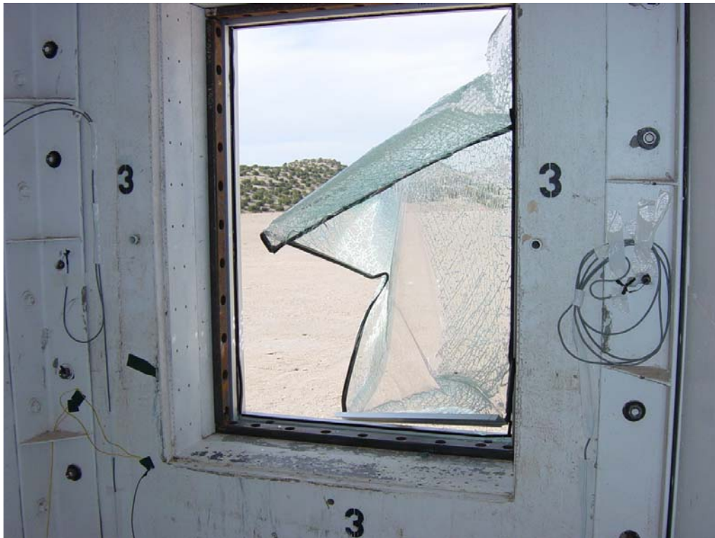
Figure 3-62 Interior post-test view of window 3. (DSC04546.jpg)
