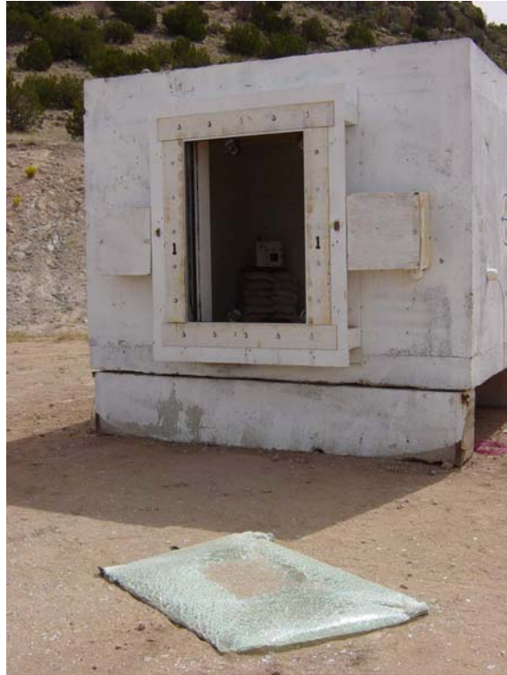
Figure 3-3 Exterior post-test view of window 1. (DSC04037.jpg)
