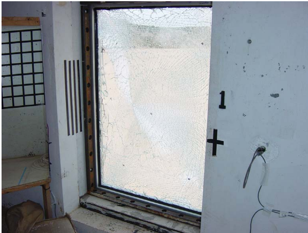
Figure 3-43 Interior post-test view of window 1. (DSC04355.jpg)
