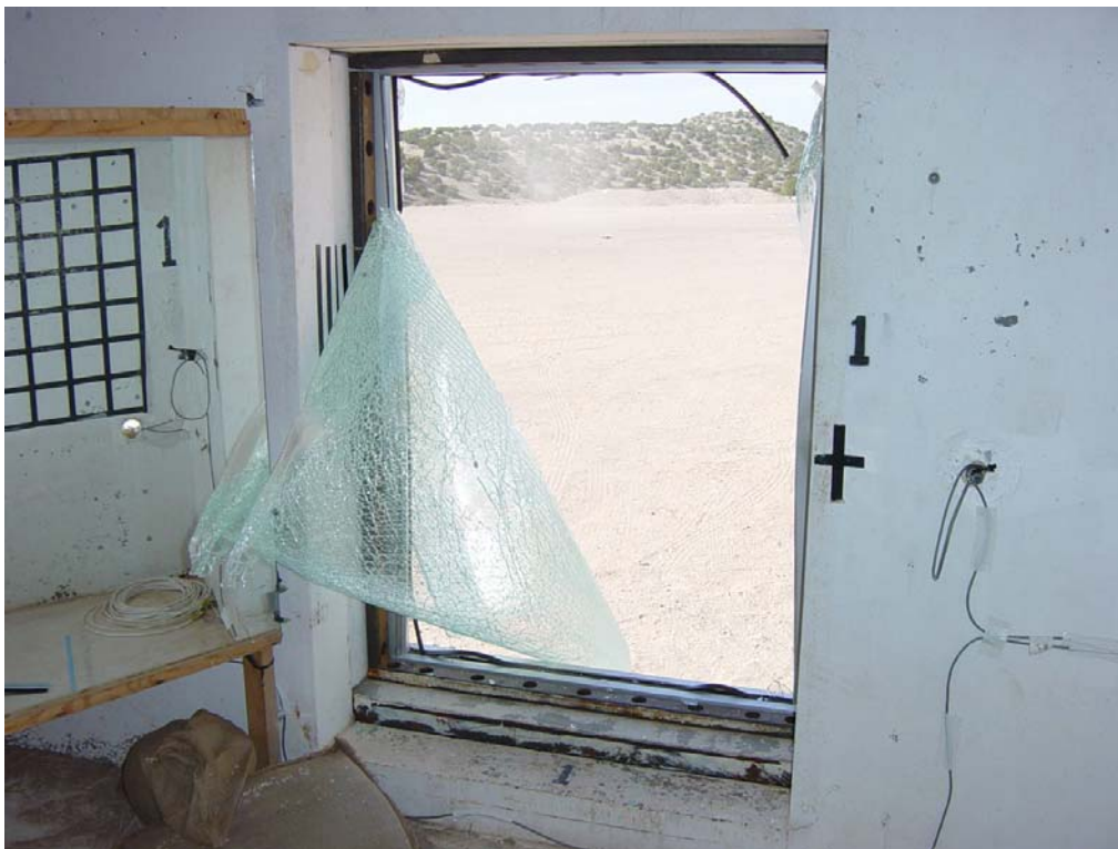
Figure 3-56 Interior post-test view of window 1. (DSC04517.jpg)
