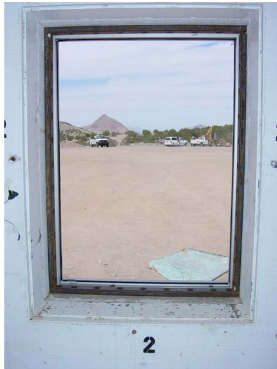
Figure 3-7 Interior post-test view of window 2. (DSC04068.jpg)
