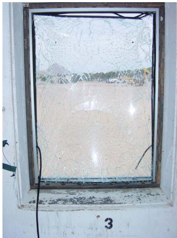
Figure 3-49 Interior post-test view of window 3. (DSC04395.jpg)
