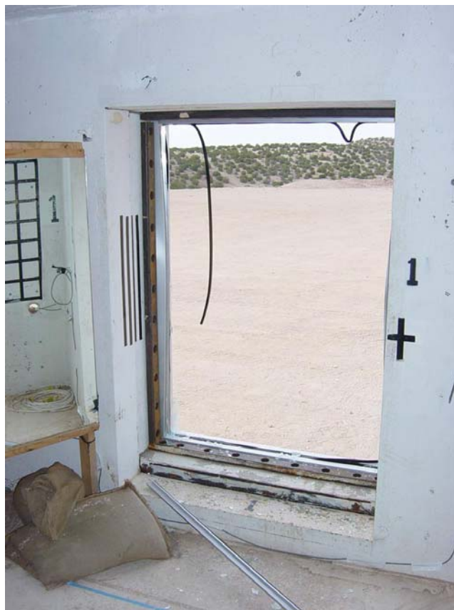
Figure 3-17 Interior post-test view of window 1. (DSC04168.jpg)
