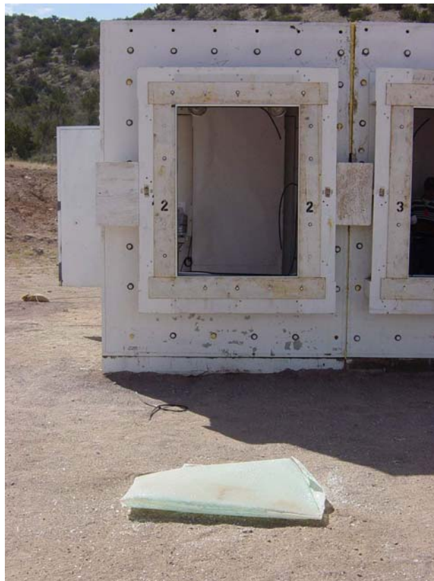
Figure 3-32 Exterior post-test view of window 2. (DSC04292.jpg)
