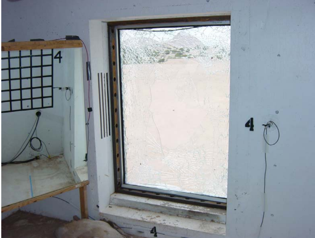
Figure 3-13 Interior post-test view of window 4. (DSC04092.jpg)
