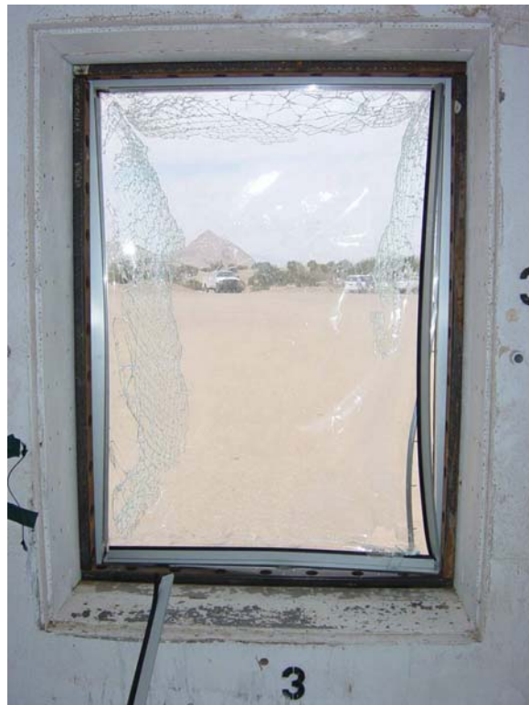
Figure 3-10 Interior post-test view of window 3. (DSC04074.jpg)
