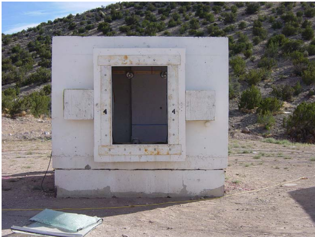
Figure 3-64 Exterior post-test view of window 4. (DSC04558.jpg)
