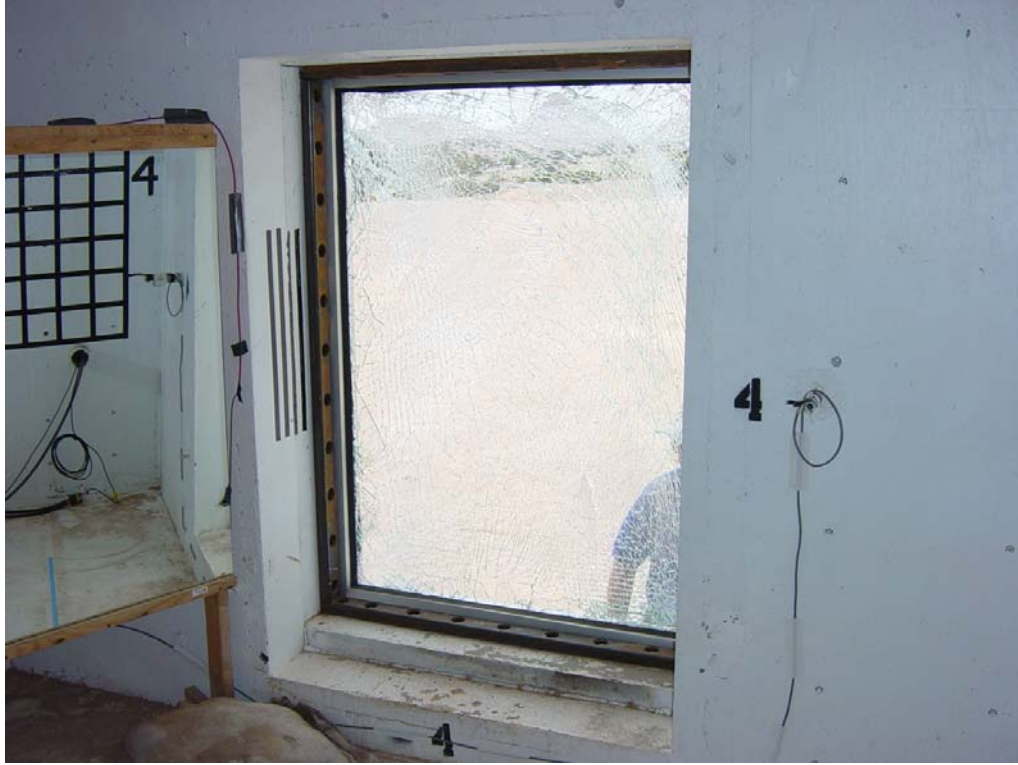
Figure 3-26 Interior post-test view of window 4. (DSC04217.jpg)
