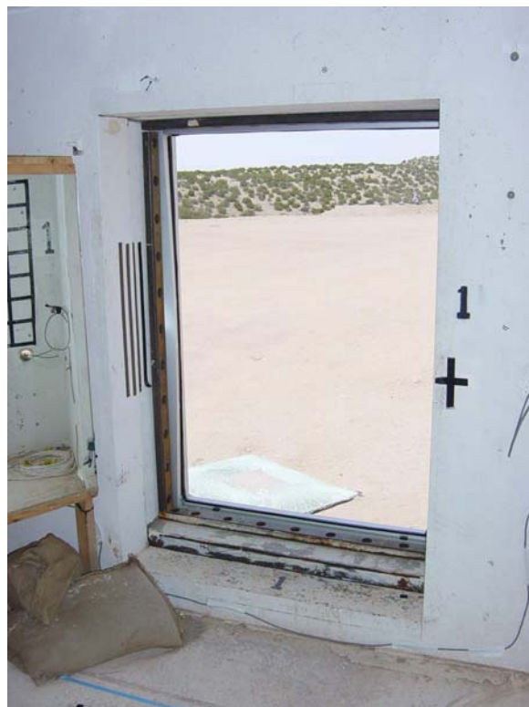
Figure 3-4 Interior post-test view of window 1. (DSC04039.jpg)
