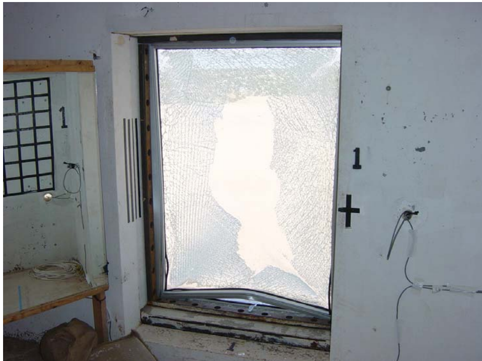
Figure 3-30 Interior post-test view of window 1. (DSC04288.jpg)
