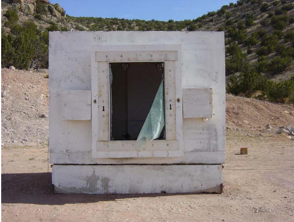
Figure 3-55 Exterior post-test view of window 1. (DSC04508.jpg)
