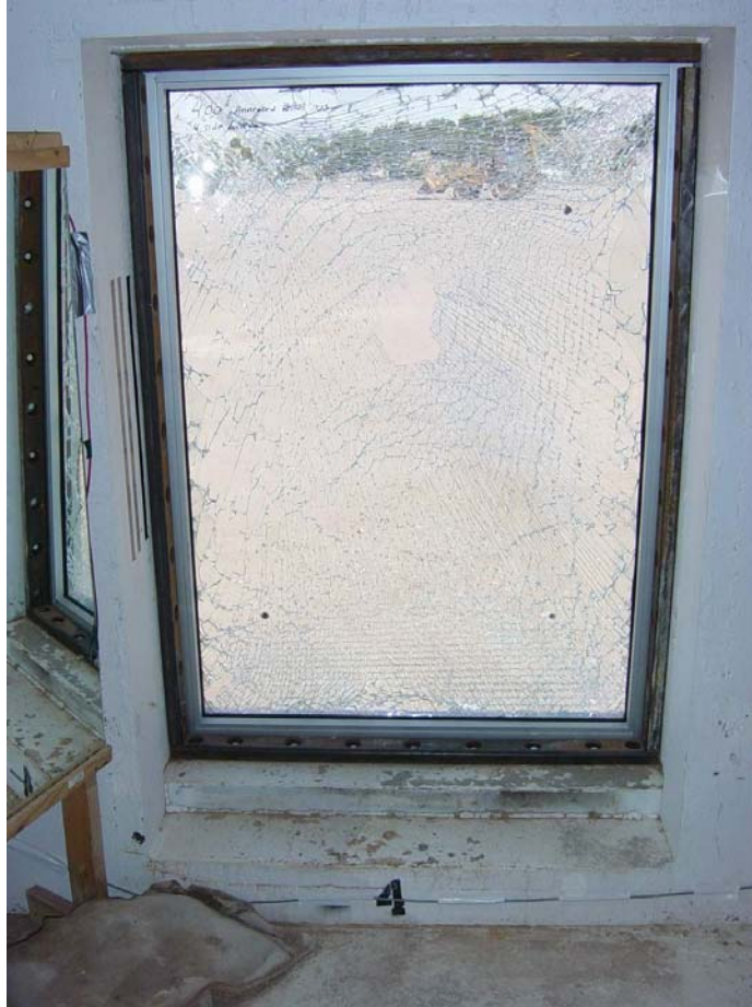
Figure 3-39 Interior post-test view of window 4. (DSC04341.jpg)
