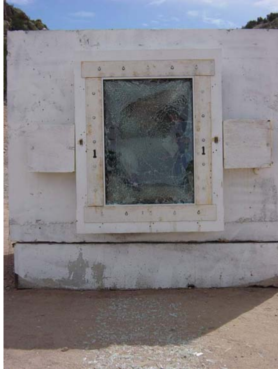
Figure 3-42 Exterior post-test view of window 1. (DSC04350.jpg)
