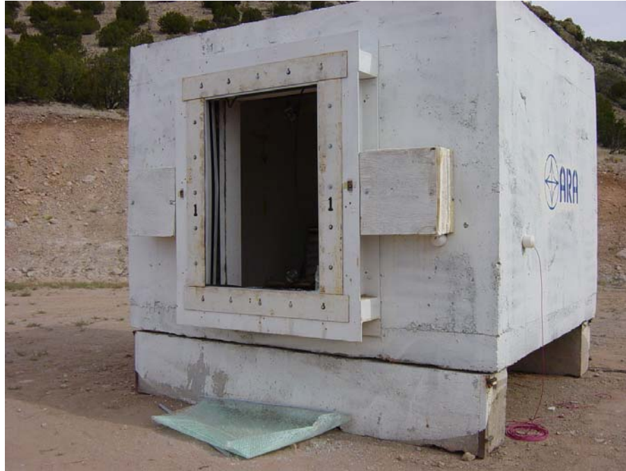
Figure 3-16 Exterior post-test view of window 1. (DSC04159.jpg)
