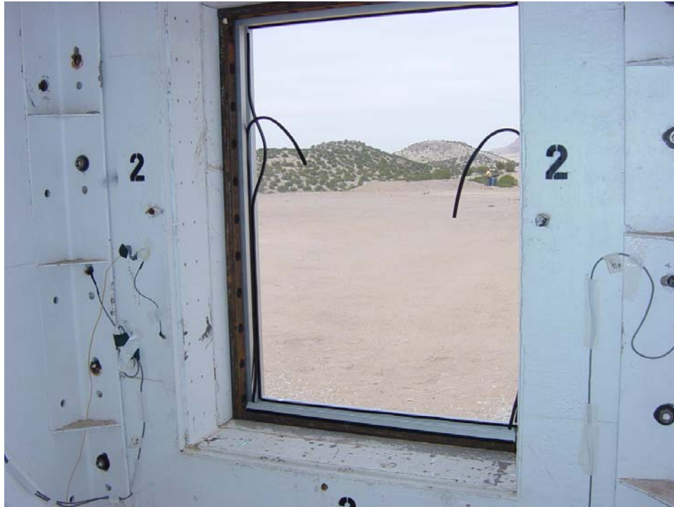
Figure 3-46 Interior post-test view of window 2. (DSC04383.jpg)
