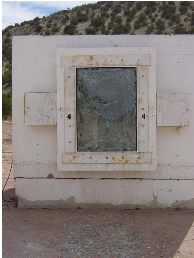
Figure 3-51 Exterior post-test view of window 4. (DSC04413.jpg)
