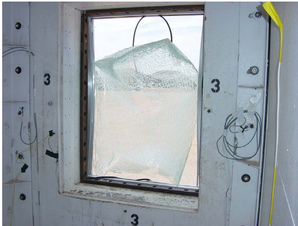
Figure 3-23 Interior post-test view of window 3. (DSC04198.jpg)
