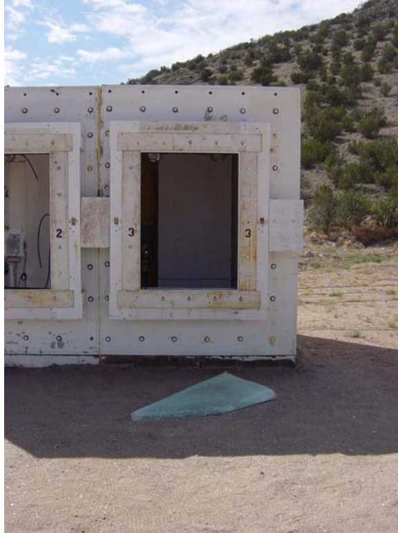
Figure 3-35 Exterior post-test view of window 3. (DSC04297.jpg)
