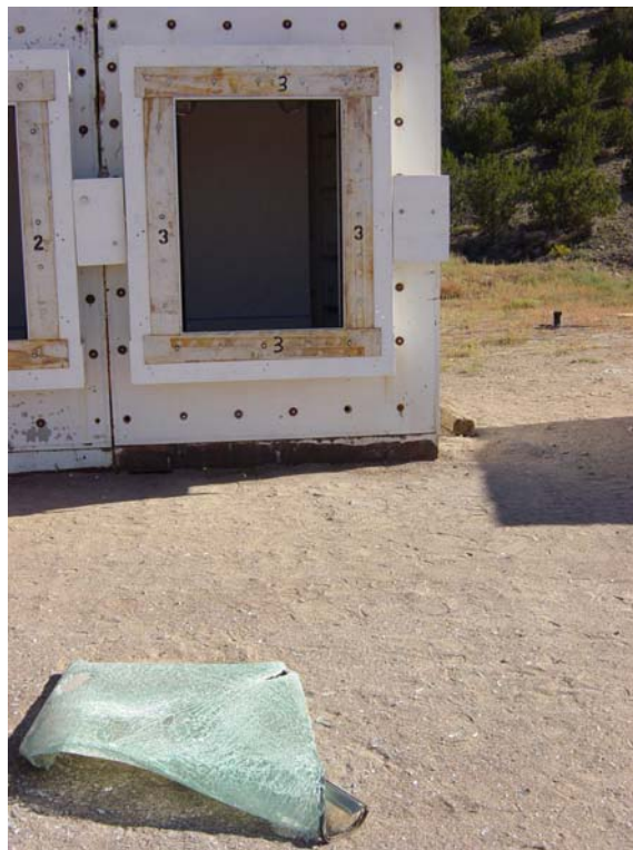
Figure 3.10. Exterior post-test view of Window 3.
