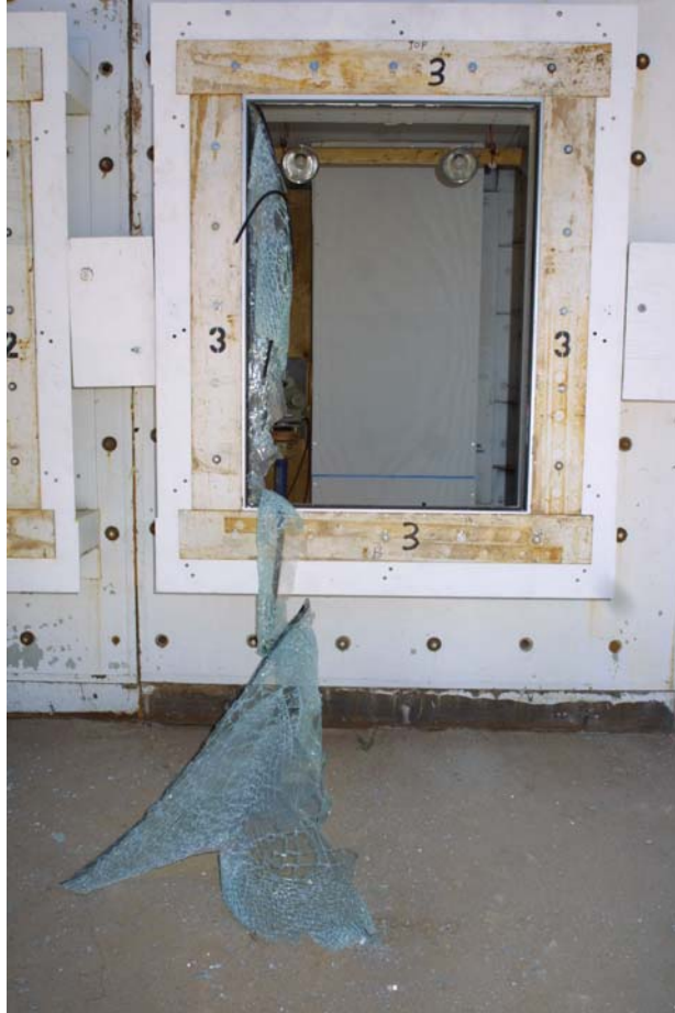
Figure 3.23. Exterior post-test view of Window 3.
