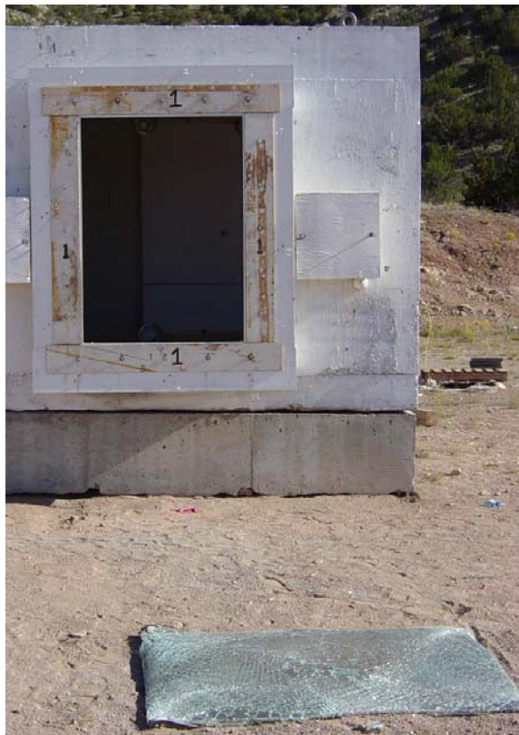
Figure 3.4. Interior post-test view of Window 1.
