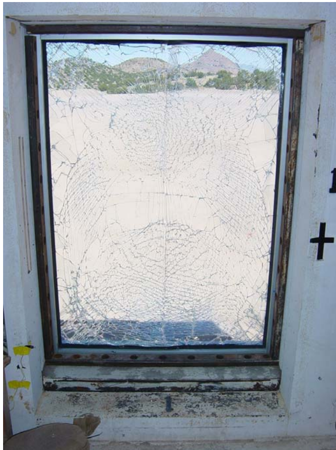
Figure 3.16. Interior post-test view of Window 1.
