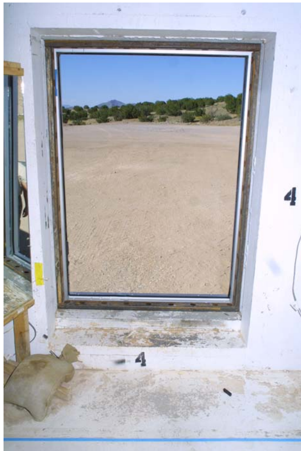
Figure 3.12. Interior post-test view of Window 4.
