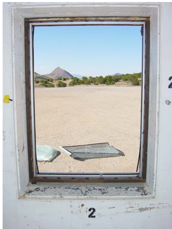
Figure 3.6. Exterior post-test view of Window 2.
