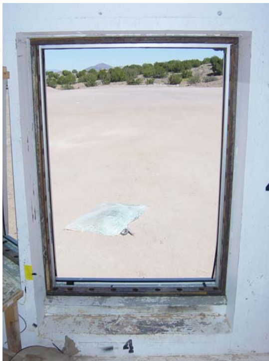
Figure 3.25. Exterior post-test view of Window 4.
