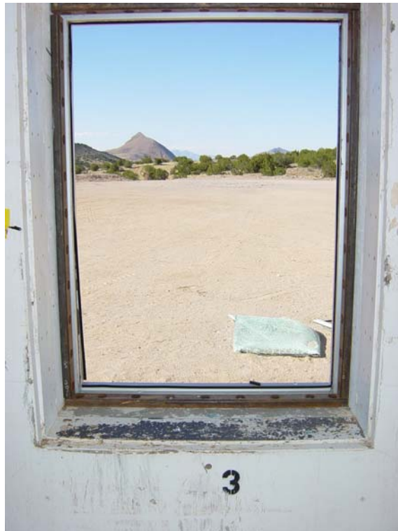
Figure 3.9. Interior post-test view of Window 3.
