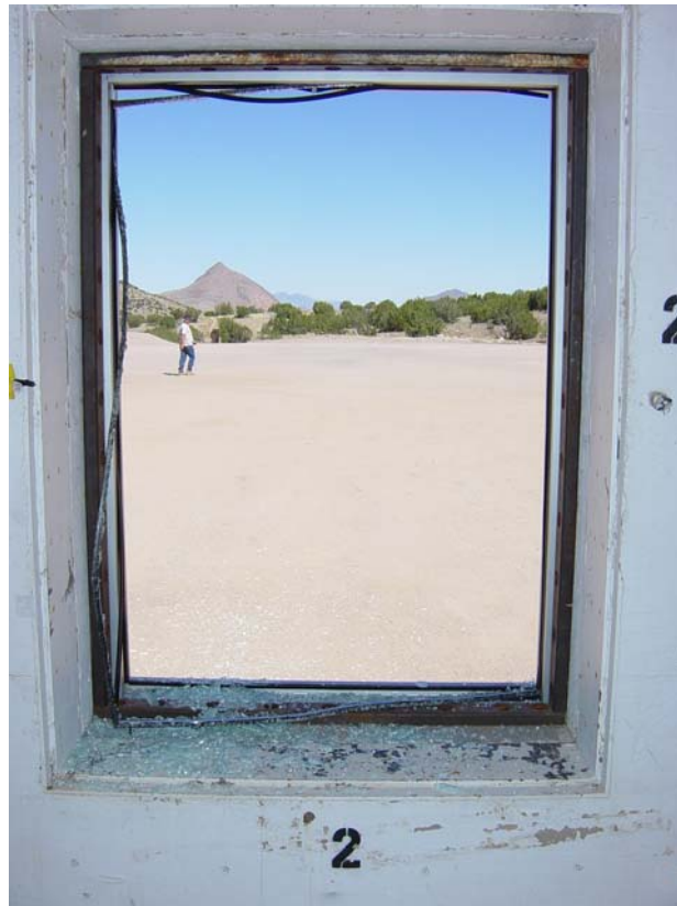
Figure 3.19. Interior post-test view of Window 2.
