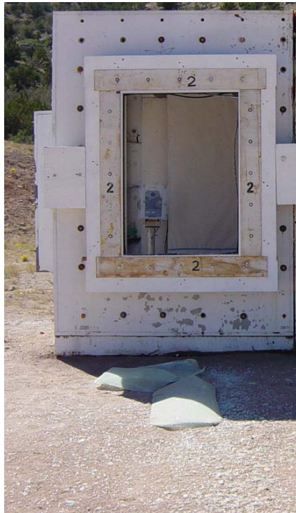
Figure 3.20. Exterior post-test view of Window 2.
