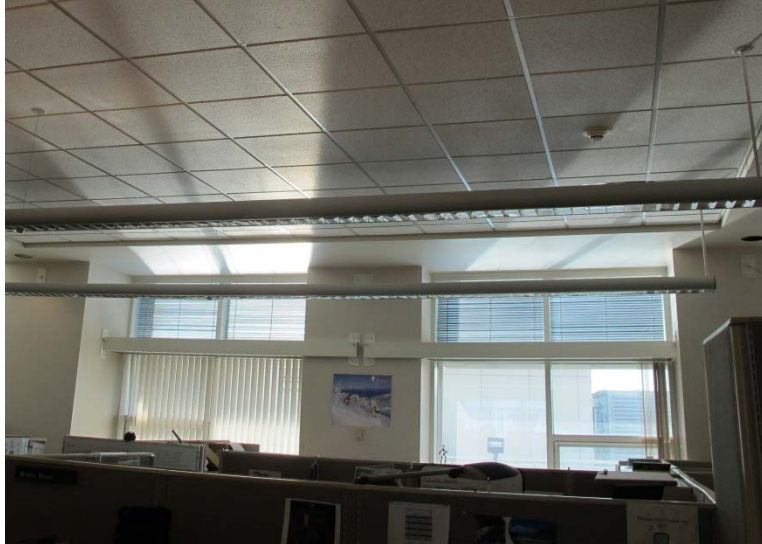
Figure 9. LightLouver™ Daylighting System installed in study area.
