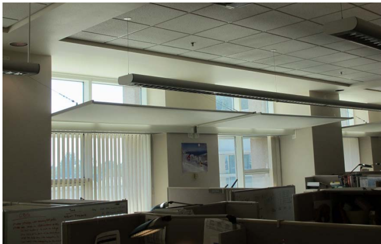
Figure 7. Light shelves as installed in the study area.
