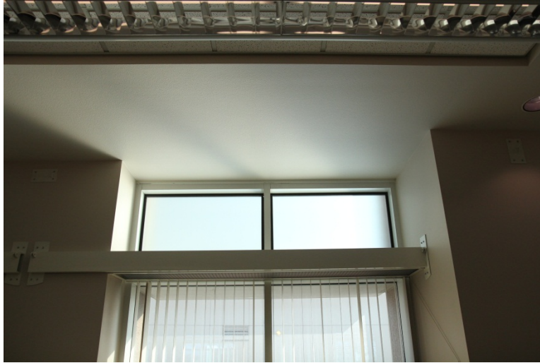
Figure 8. 3M's Daylight Redirecting Window Film installed in study area.
