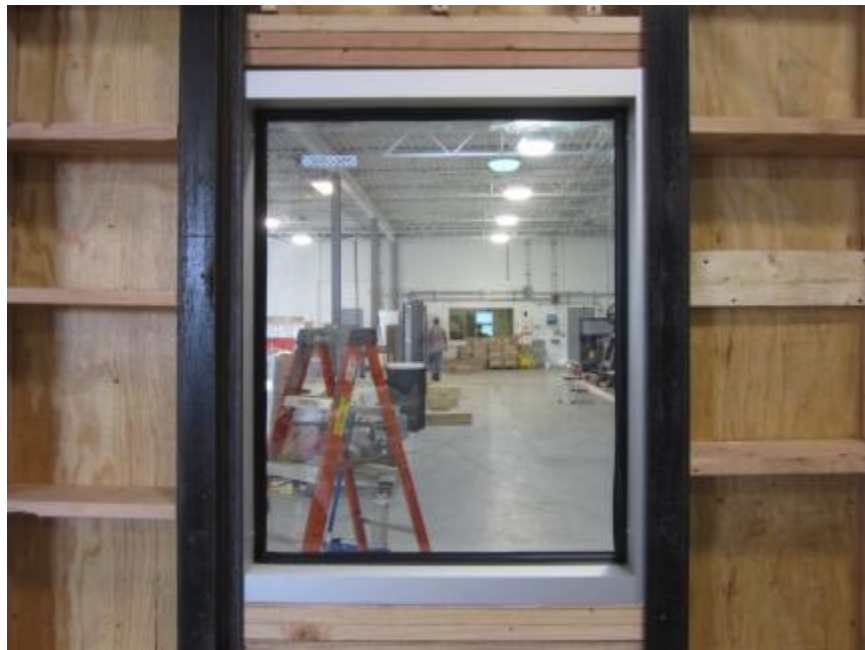
Photo No. 10 Pre-test Specimen #4, Interior
